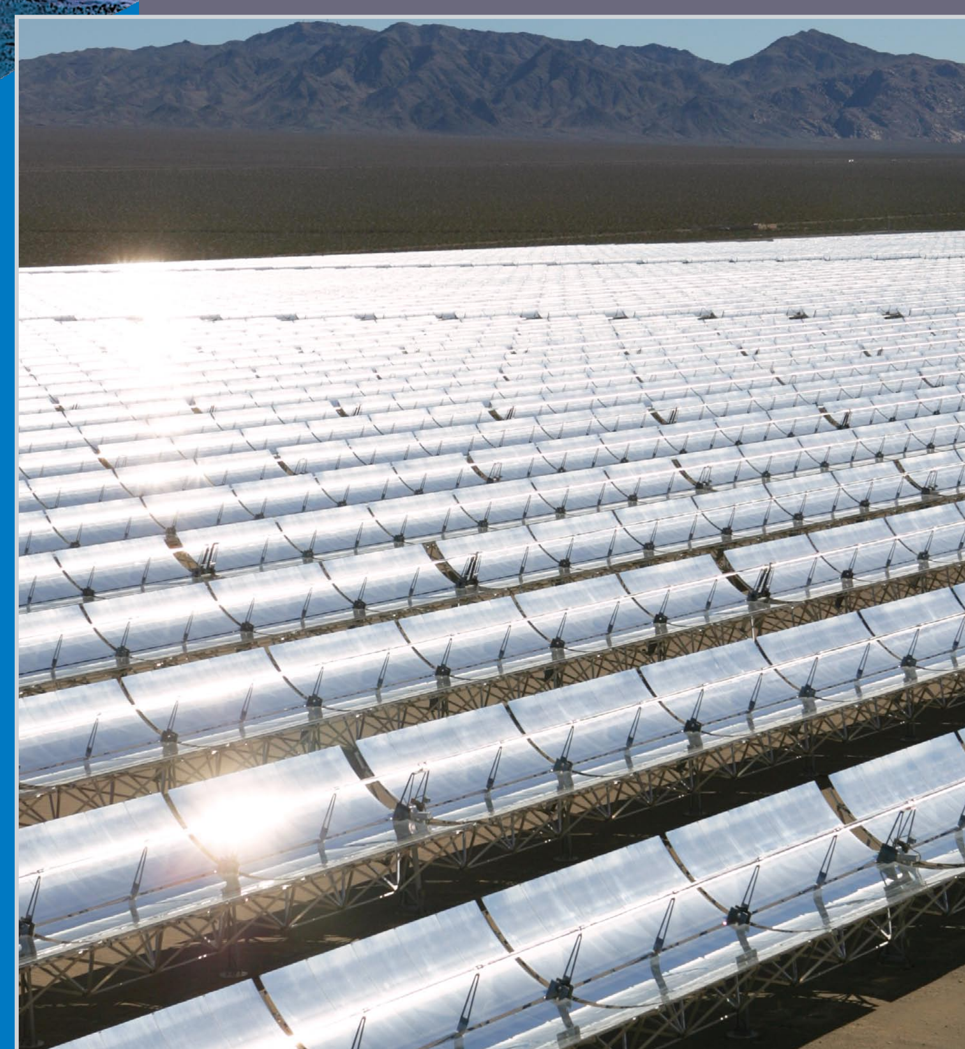
A section of the parabolic troughs from the Nevada One project tracking the sun.
