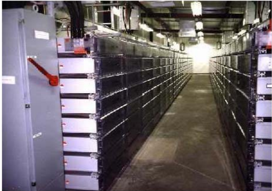
A 5-MVA battery energy-storage system for power quality and peak shaving.
